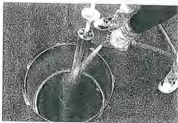
Photo 2. Spray the cartridge tubes with a hose.
