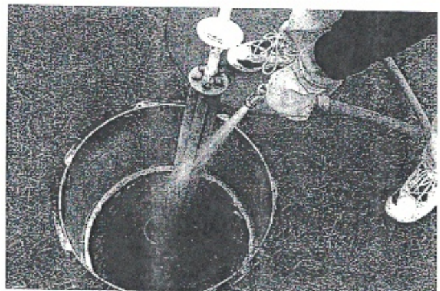
Photo 2. Spray the cartridge tubes with a hose.
